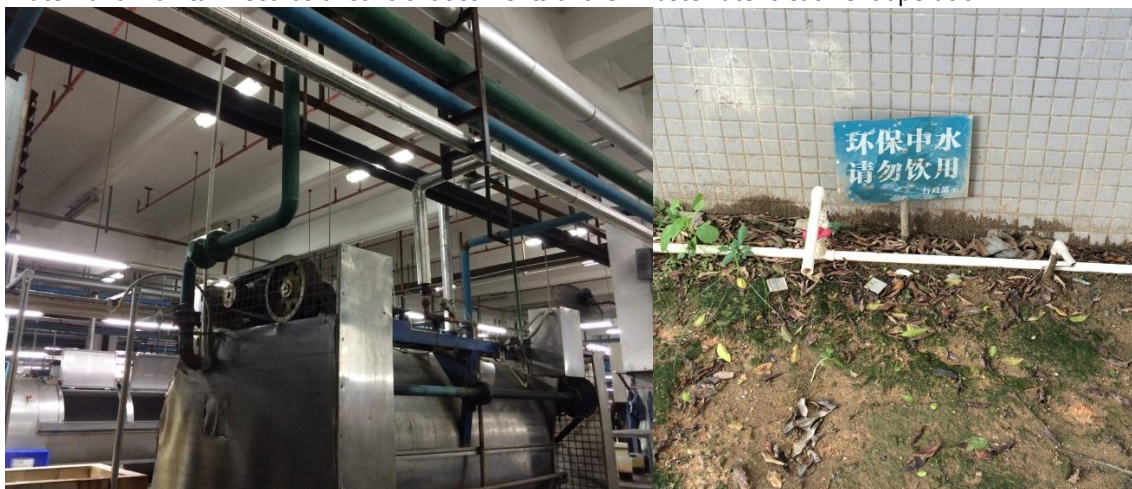
Figure 14: Preventative measures at the Yida Facility; Color coded piping shows fresh water (blue pipes) and recycled water (green pipes) connecting to each machine (Left) and “Do Not Drink” warning sign (Right)
