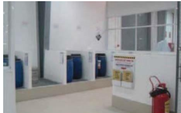
Good Practice: Chemicals stored in designated area. Area is clean and housekeeping is good.
