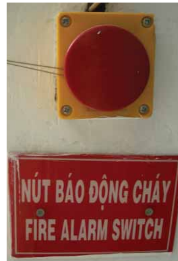
Good Practice: Fire alarm switch in native language.
