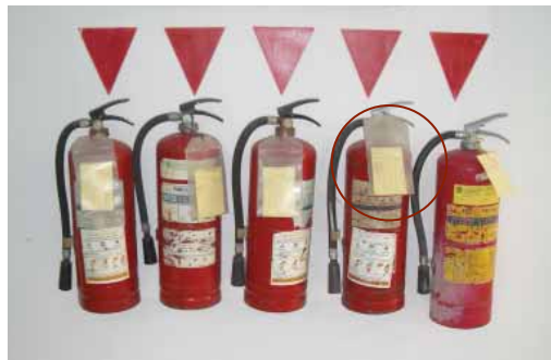
Good Practice: Fire extinguisher types for potential hazards are provided and tagged.
