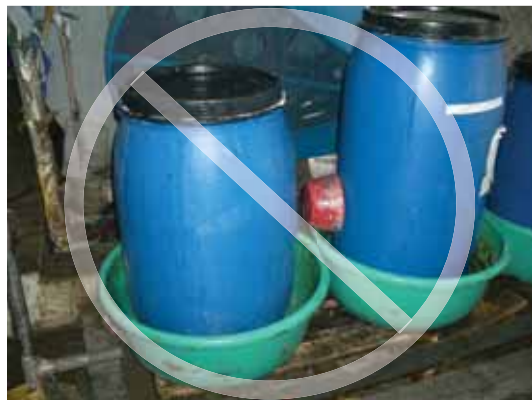
Bad Practice: Secondary containment is too small for these chemical drums!
